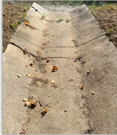
Figure 4. Example Photo showing cracking of a concrete flume.
